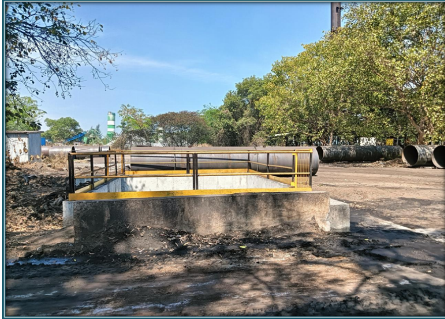
Rainwater Collection pit at CPP II coal yard
