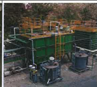
Rapid Clarifier System
