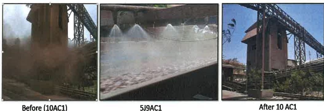
Dust suppression nozzles for JH 9A - RMHS
