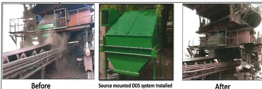
Source mounted dedusting units for SR4 - RMHS
