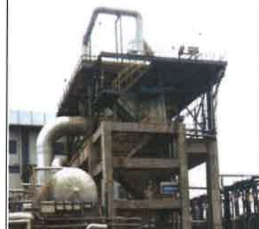
Multiple Effective Evaporator for ZLD plant
