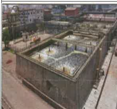
MBR+RO+ZLD plant at Coke Oven (4000 m3/d)
