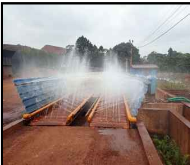
WHEEL WASHING SYSTEM
