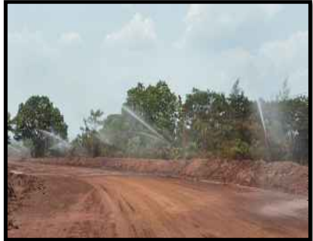
FIXED WATER SPRINKLER
