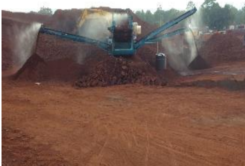
Dry Fog System in Mineral Handling Plants
