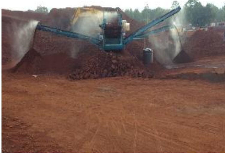
Dry Fog System in Mineral Handling Plants
