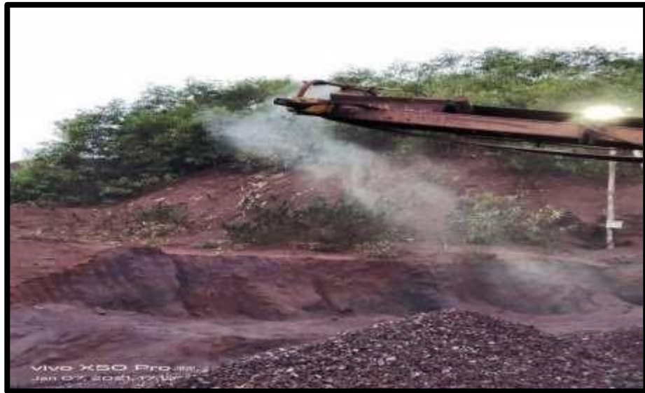
Dry Fog System in Mineral Handling Plants
