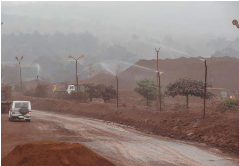
Fixed Sprinkling System
