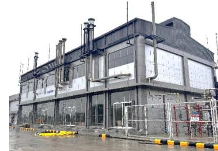
Green Hydrogen Electrolyser at Vijayanagar
