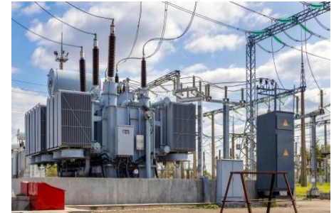
Electric Power Transformers
