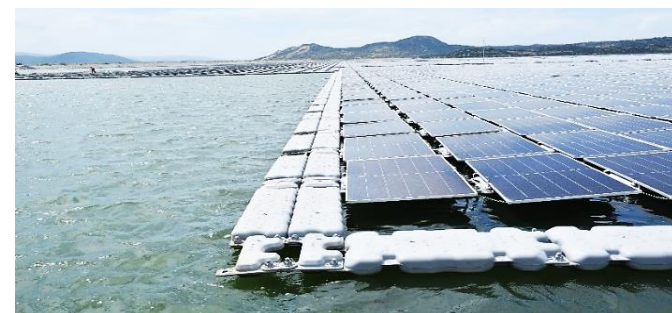
20MW Floating Solar Project at Vijayanagar, Karnataka
