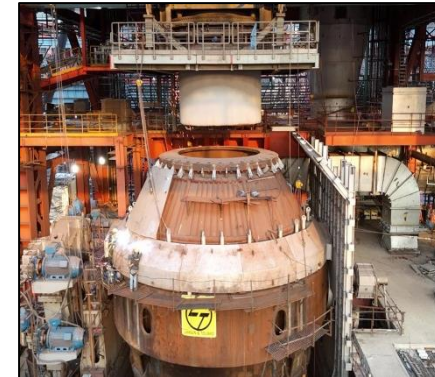
Converter-2 at SMS
