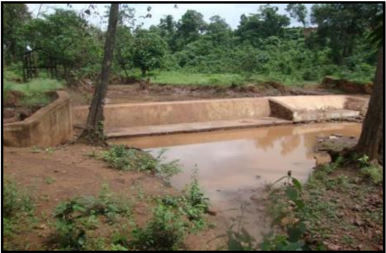
Check Dam Provided at Topadihi Nalla Nalla Side Plantation
