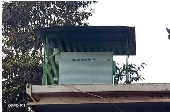
Online Noise Monitoring Device
