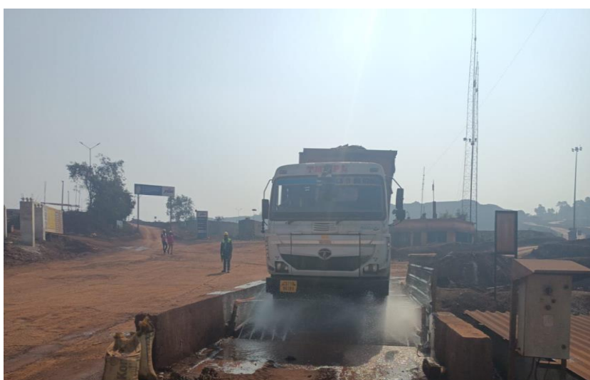
Mechanised wheelwashing System
