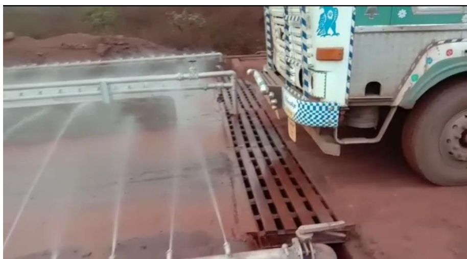
Wheel Washing System near Gate No 6.
